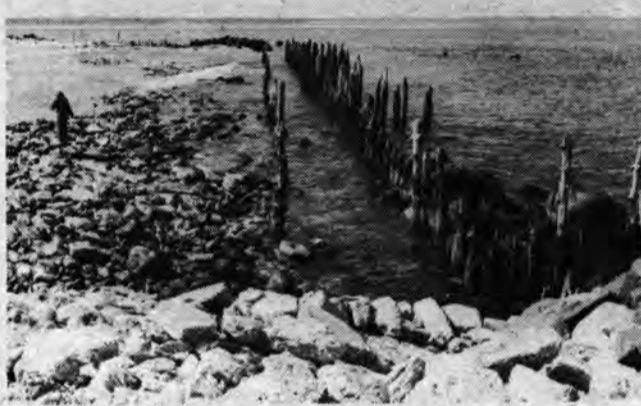
Jetties ready to collapse at Shinnecock
