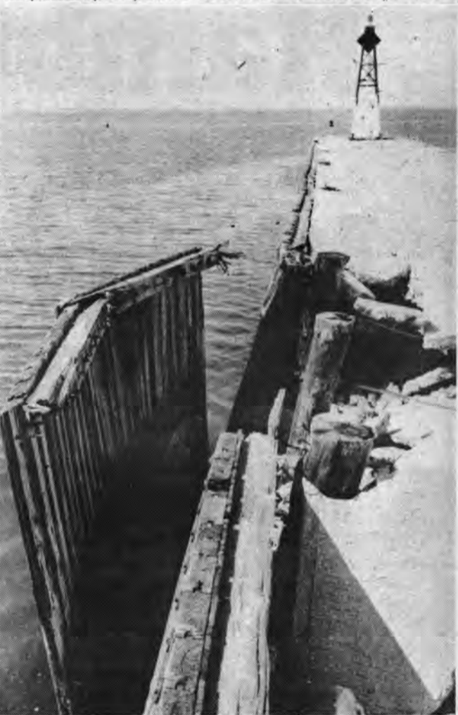
County-owned bulkheading that is falling apart
