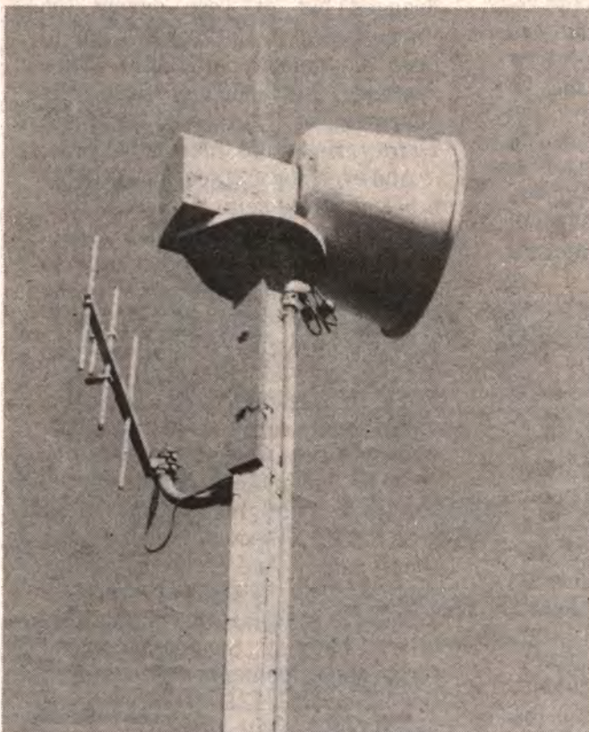
SIRENS SOUND AGAIN--Long Island Lighting Company officials tested the Shoreham emergency sirens again last week, reporting that 87 of 89 worked properly. The testing came shortly after a federal court ruling upheld the Nuclear Regulatory Commission's rule change on evacuation plans. Photo by Jeff Sievers. (Full V48F)
